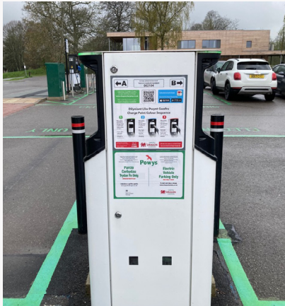
Example of EV Charge point
